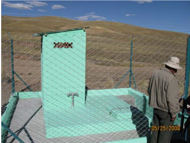
Storage tank – Huallitiri
