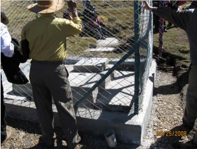
New storage tank
