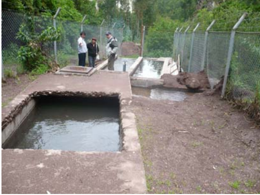
Surface water diversion structure in need of modifications, community of Yucay, in the Urubamba River Valley
