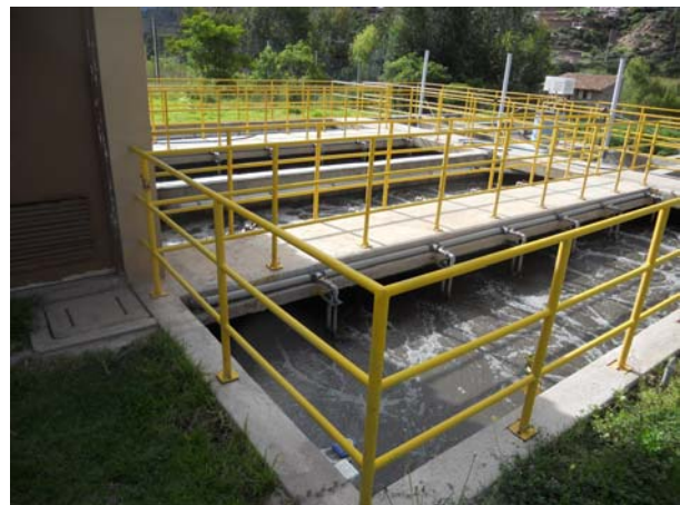
Hotel 'Tambo del Inca' wastewater treatment plant
