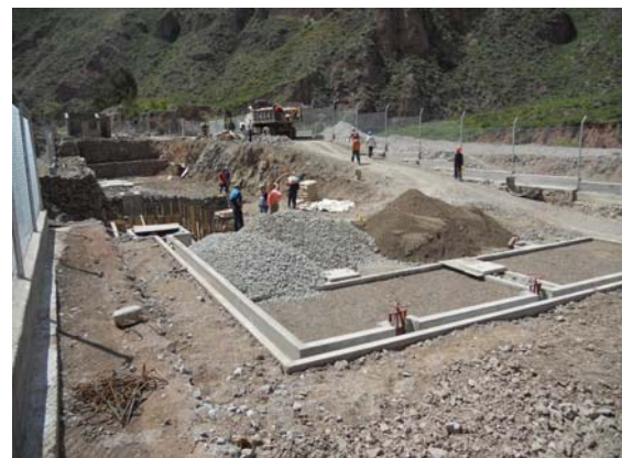
Pumahuanca treatment site with sludge drying beds
