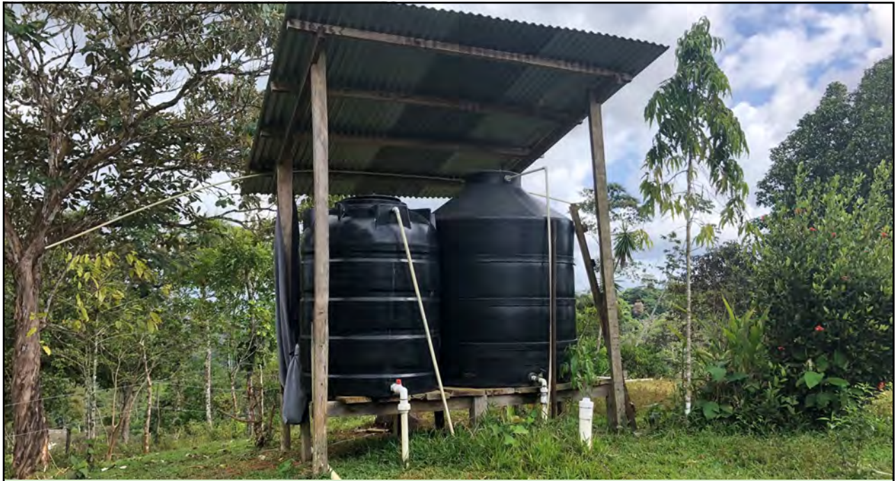
Guayabo: Water supply tanks
