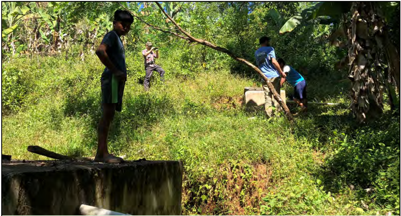
Quebrada Pavo: WEFTA team reviewing the storage tank site and sedimentation tank.
