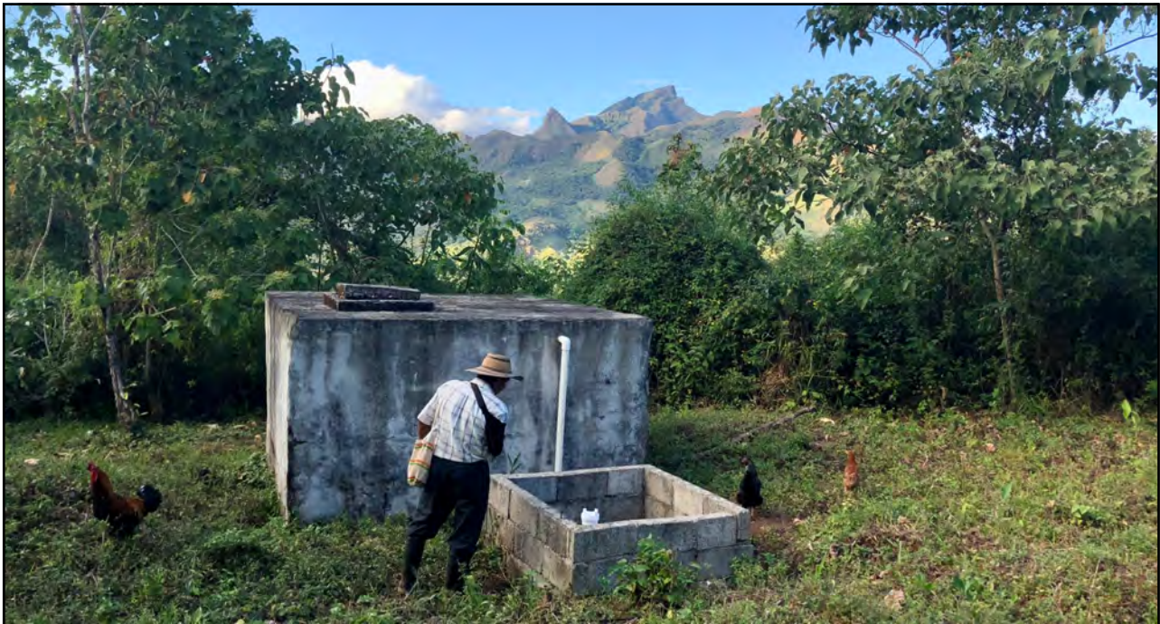
Alto Estrella: WEFTA team reviewing the tank and chlorinator
