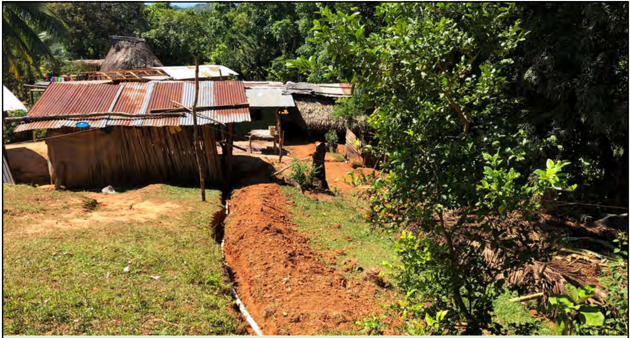
Quebrada Pavo: the community is still working to bury all pipes from the project.
