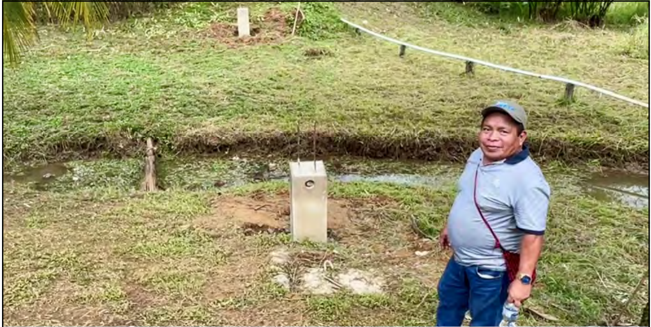
José Molina, WEFTA's In-Country Project Manager for Bocas del Toro is a proud WASH system contractor. Here he poses with the initial columns for the bridge to provide the water transmission line a safe creek crossing.
