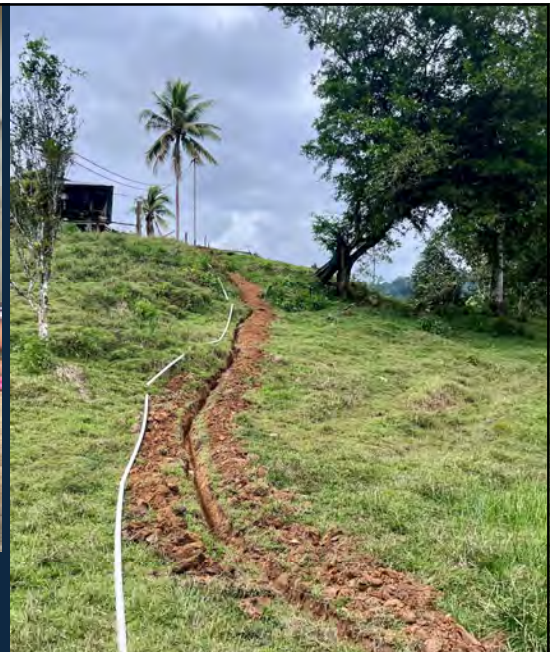
The community of San Martin has made exceptional progress with the improvements and expansion of their WEFTA - funded system.
